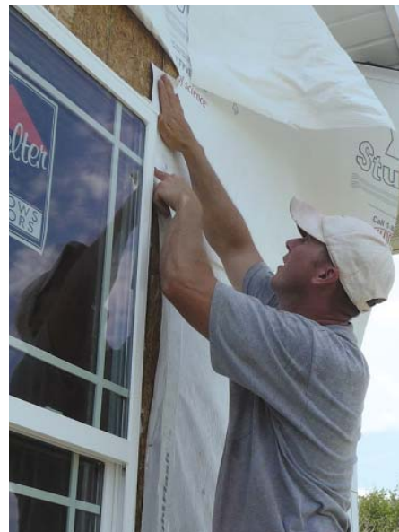
Figure 2. A sill pan fashioned from FlexWrap (far left), installed on top of the StuccoWrap, protects the rough window opening. The window is reinstalled with the nailing flanges set in sealant, then taped to the StuccoWrap (left).
